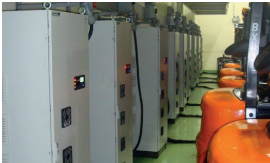
Access 400 chargers built up of Access 100 modules, 80 V 400 A, batteries 930 Ah
