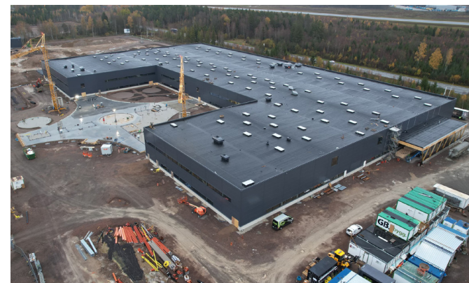
Phase 2 – Production for Lithium-ion batteries. Picture from fall 2023.
